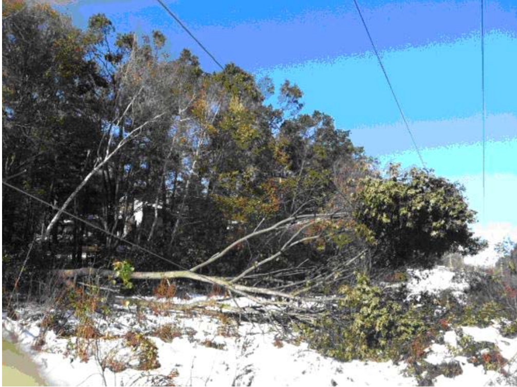
Figure 13: Trees Fallen on 115kV Line in Connecticut
