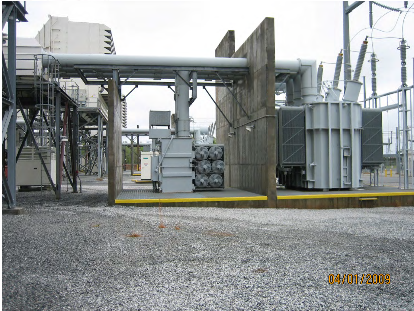
GSU Transformer, Auxiliary Transformer and Isolated Phase Bus
