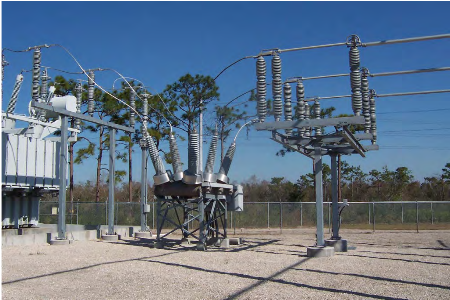
HV Substation Breaker
