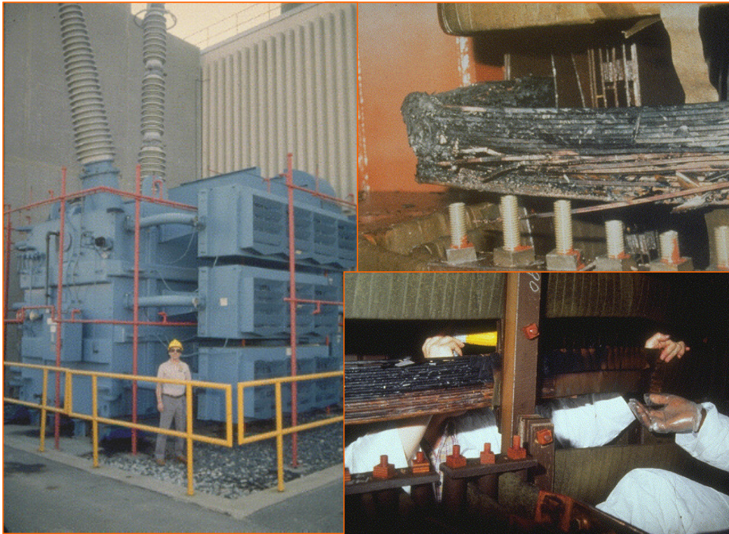
Figure 2-33. Damaged transformer at the Salem Nuclear Plant.
