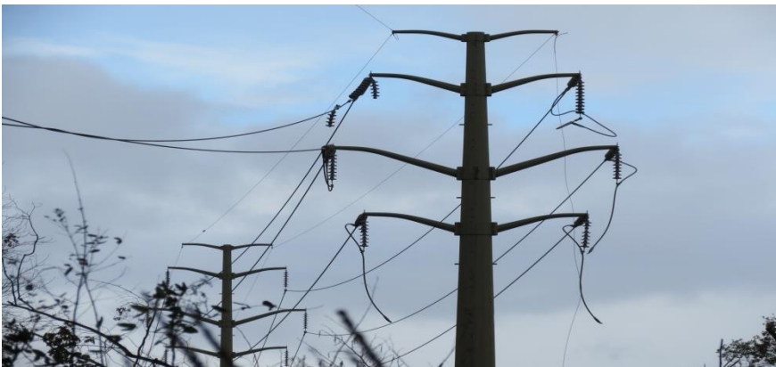
Damaged high voltage transmission line
