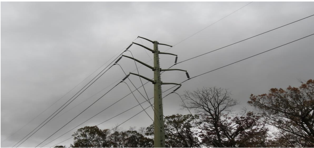
Damaged high voltage transmission line
