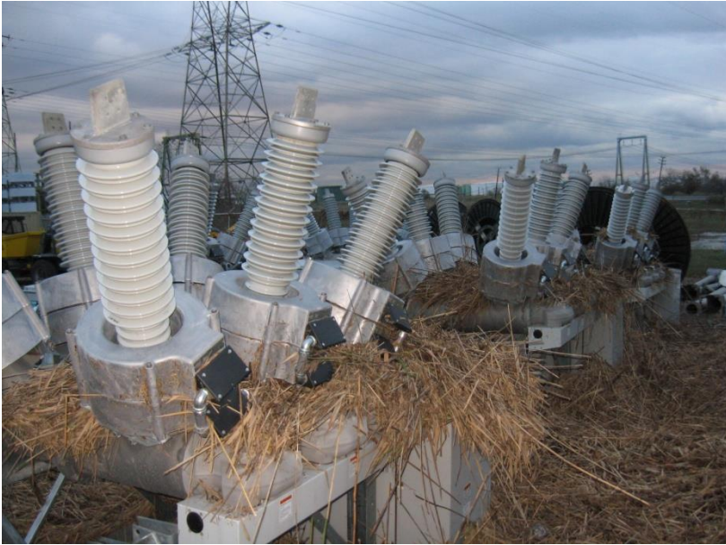
Damaged substation equipment
