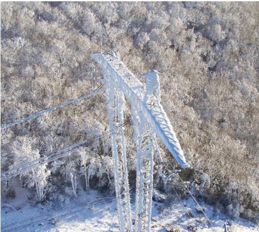
Workers hooked a crane truck to a bulldozer and pulled it more than seven miles past the nearest road to reach this transmission structure on top of East River Mountain near Bluefield. The then used the crane to place a downed static wire back on top of the snow-covered structure.
