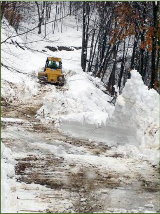
Crews had to clear more than three miles of road through remote terrain to access and repair a line.
